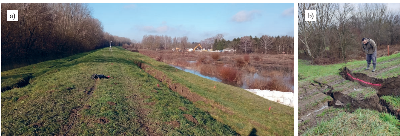
Figure 7. Subsidence and lateral spreading of the embankments near the Sava river: a) in Sisak (observation point Si-03); b) in Palanjek (observation point NP-21).
