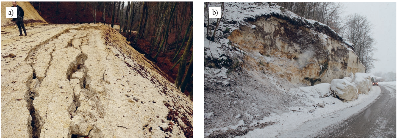
Figure 8. Coseismic landslide activation: a) slide in forest road embankment (near Strašnik, observation point ŠP-3); b) rockfall near Pecki that blocked the local road (observation point IK-ODR).
