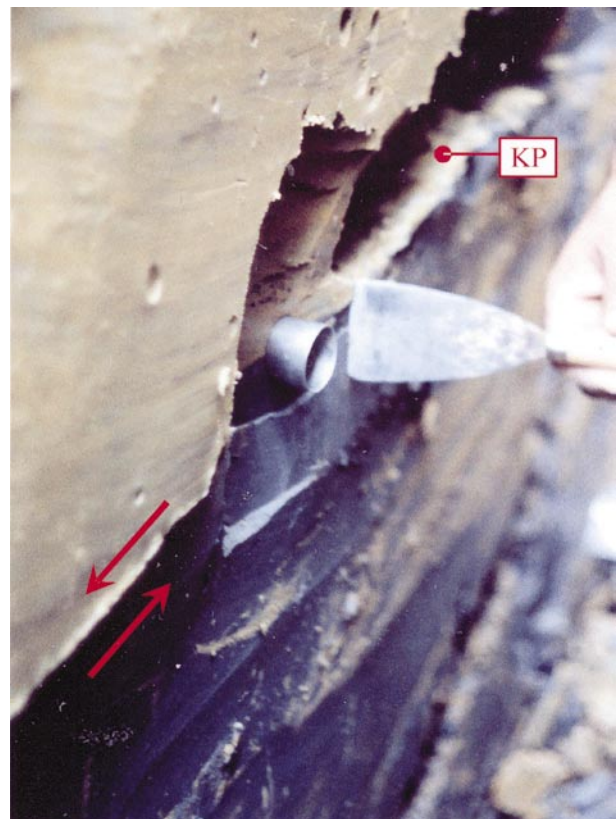
Fig. 6 Sampling in the immediate vicinity of the slip plane (KP) in drain "6" (Photo by V. Belošević, May 7, 1998).
